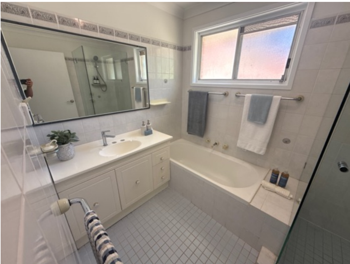
The ground floor common bathroom area tested for leaks, was issue free at the time of inspection.
