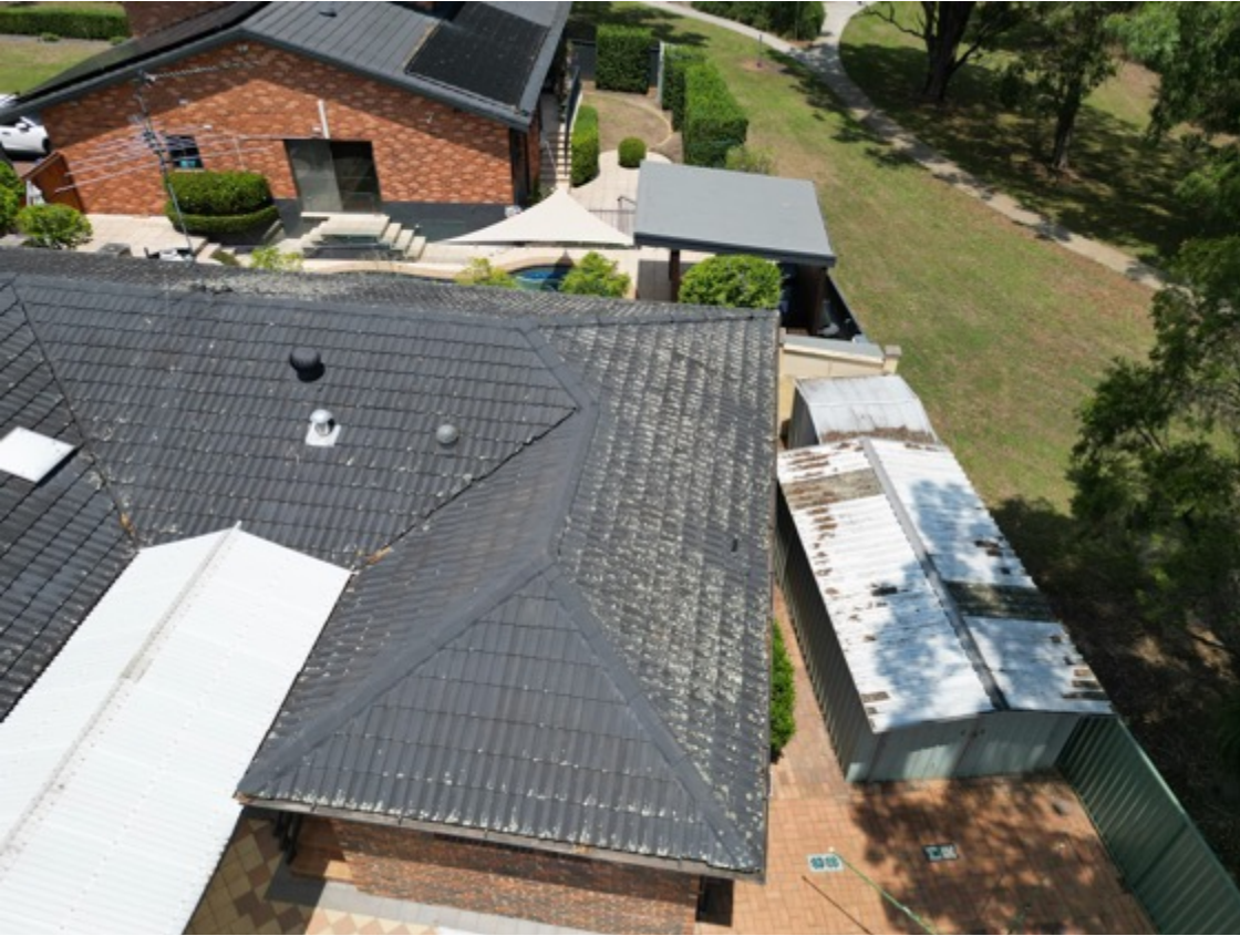
Isolated sections of roof tiles are chipped, consistent with age.
