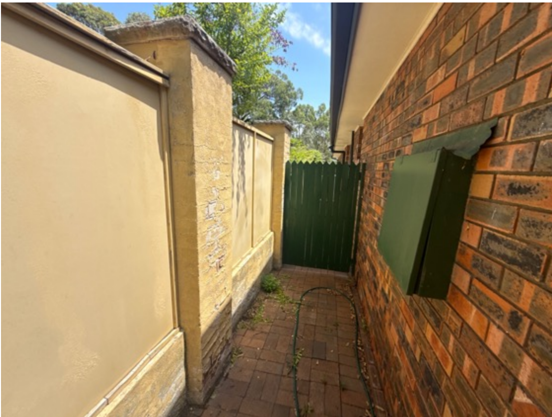
Site retaining wall render is peeling.
