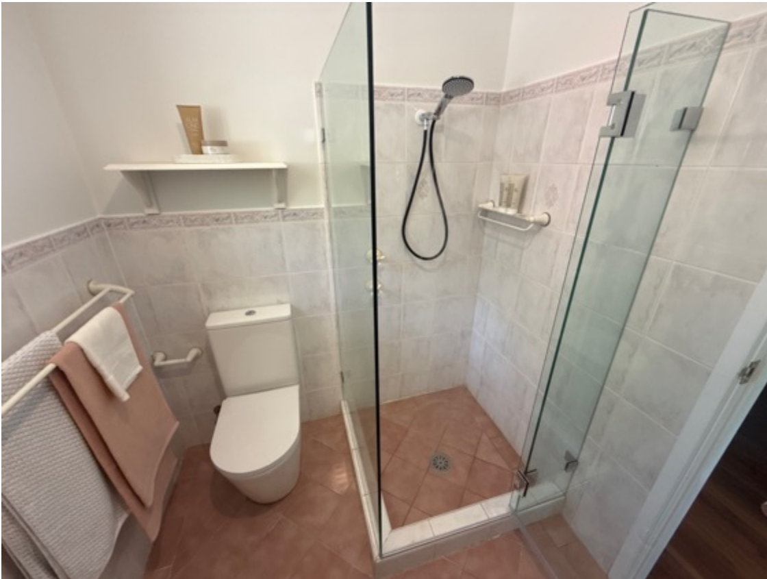
Hot and cold water services tested, functioned as intended at the time of inspection.
