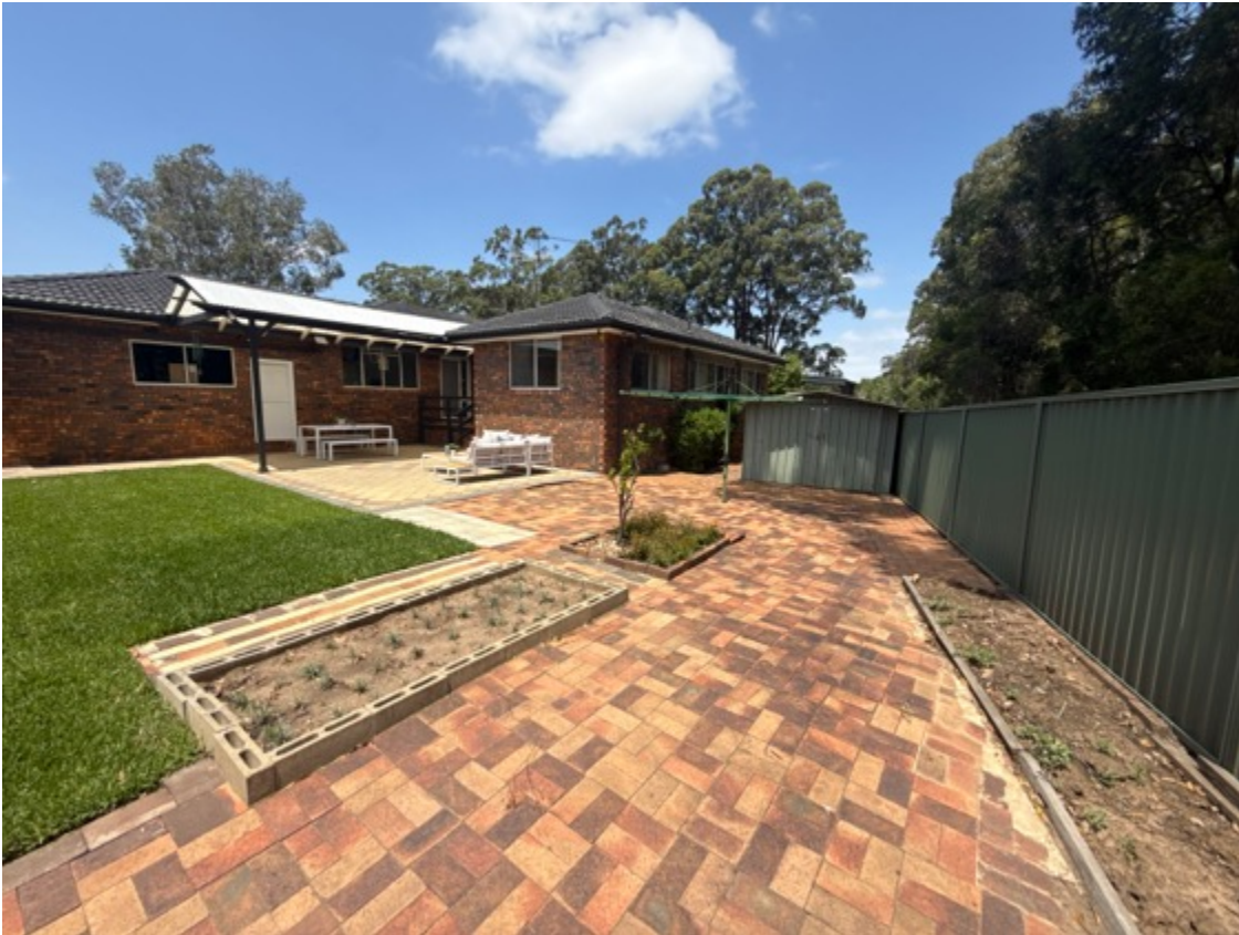
Exterior pavers present in satisfactory condition for the age, isolated sections are cracked and undulating (consistent with age.)
