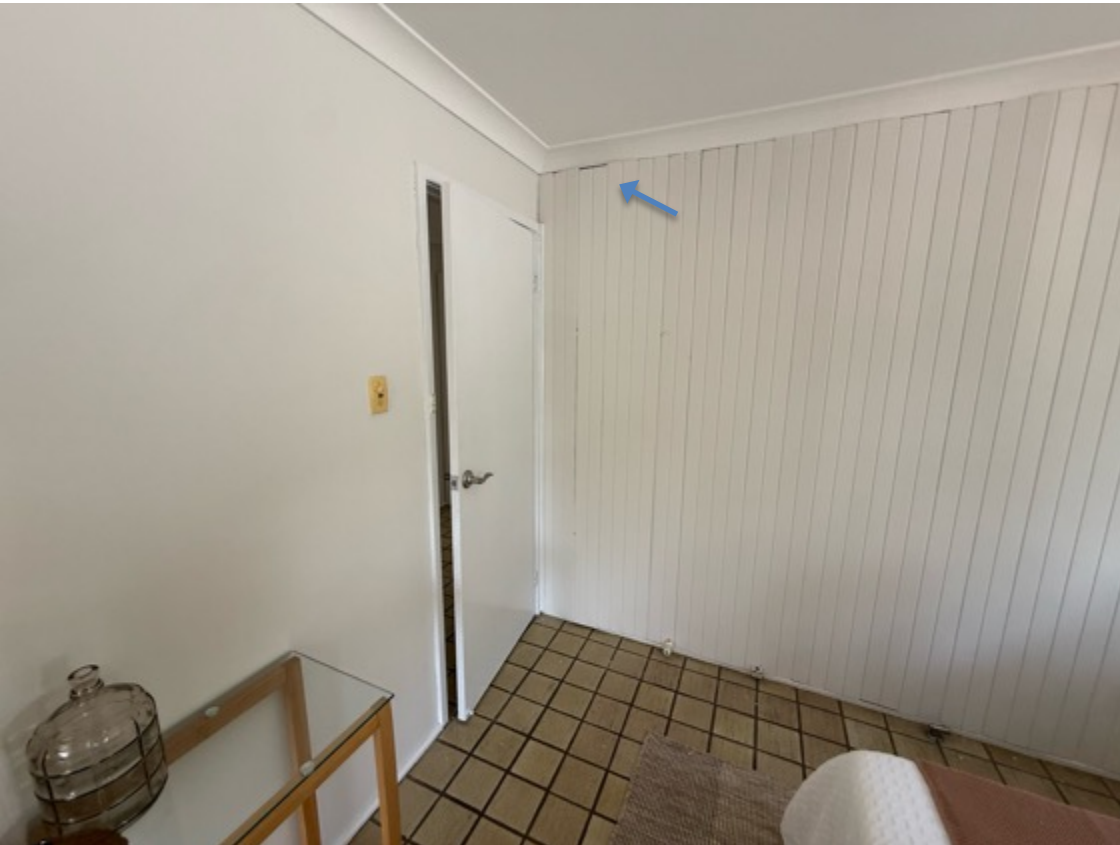
Rear bedroom wall panelling requires remedial works.
