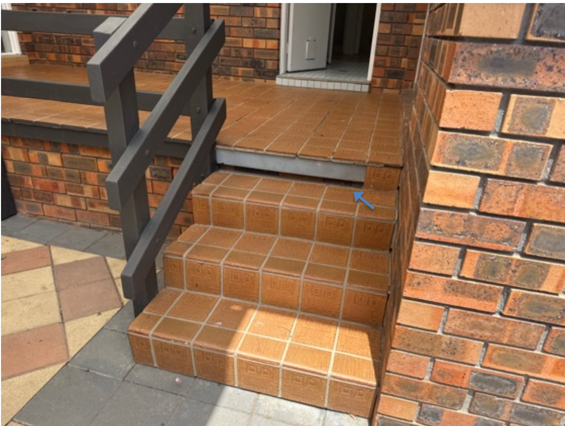
Isolated sections of tiles are cracked and display separation - there is no step to the rear of garage access door.
