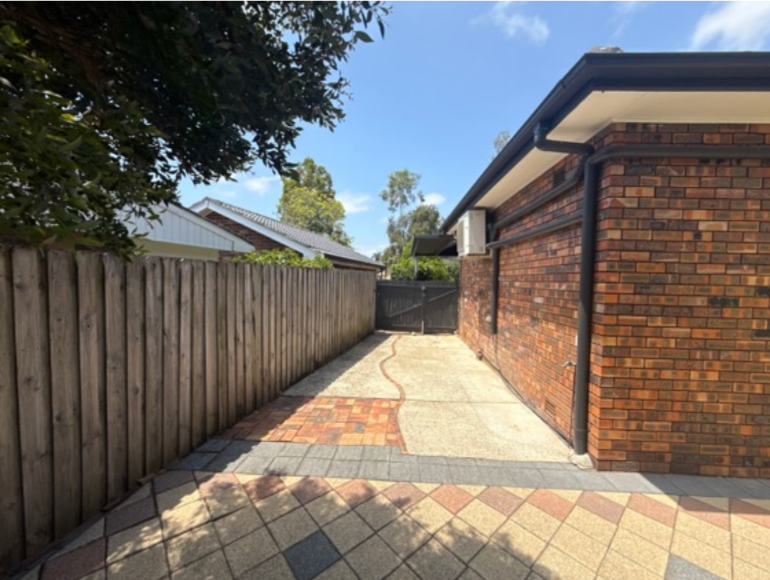
Site fences are in serviceable condition, display moderate level weathering – consistent with age.
