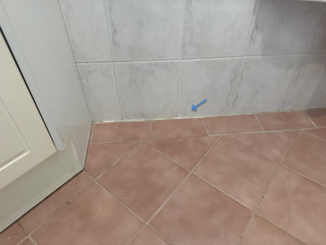
Isolated sections of tiles are cracked, consistent with age.
