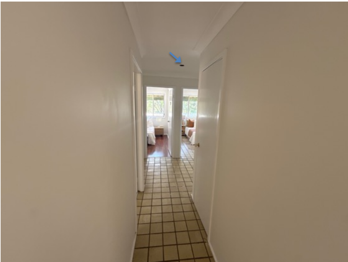
One bedroom hallway downlight is missing.
