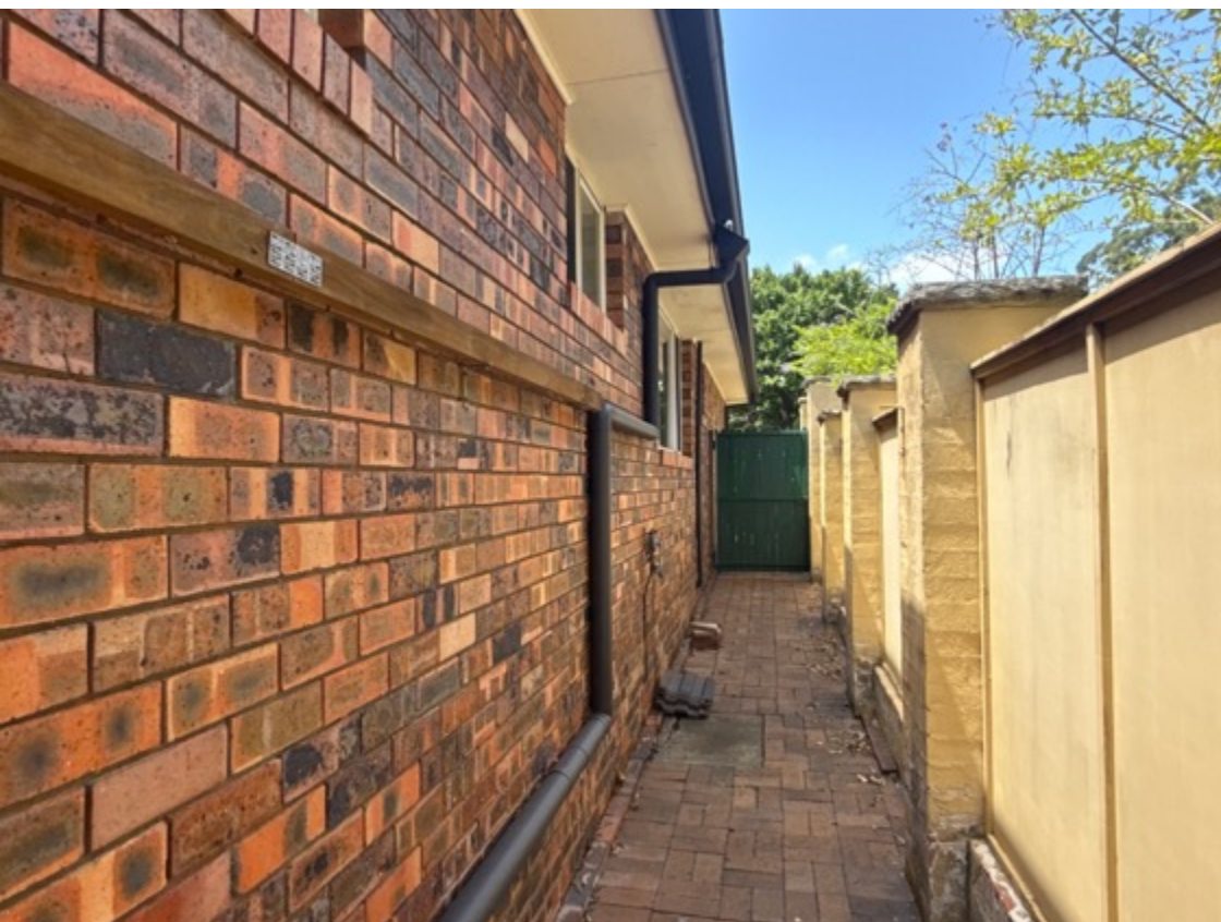
Exterior surfaces display moderate level paint blemishes, eaves lining example above.
